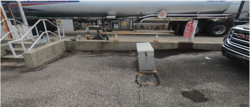
FUEL FARM B OFFLOAD CONNECTION
