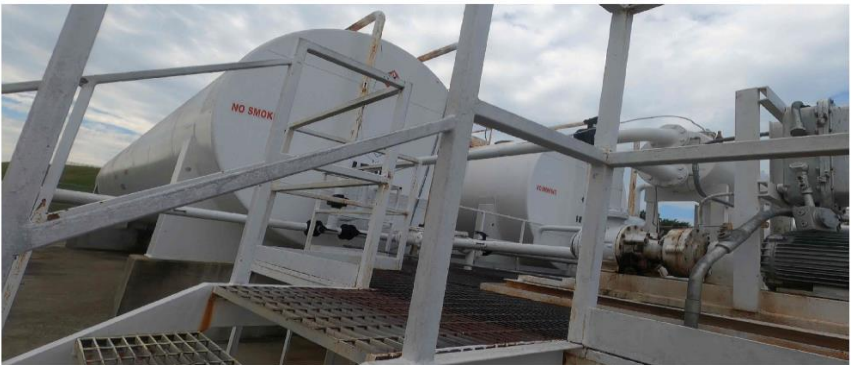
FUEL FARM B PUMPS AND FILTER SEPARATORS
