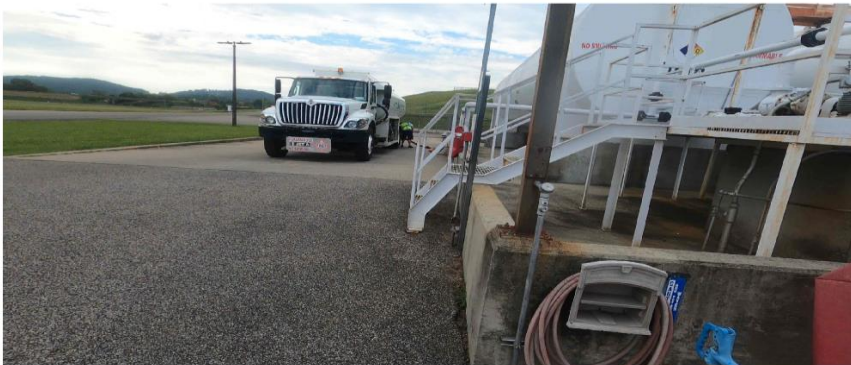
FUEL FARM B LOADING RACK
