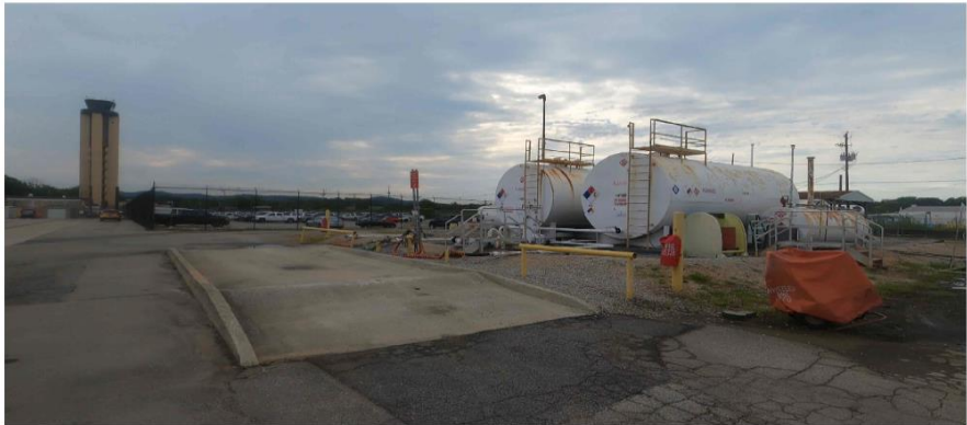
FUEL FARM C LOADING RACK
