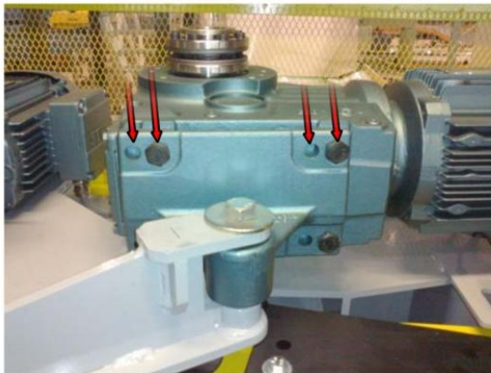
Figure 20 Wrong positioning of bolts
