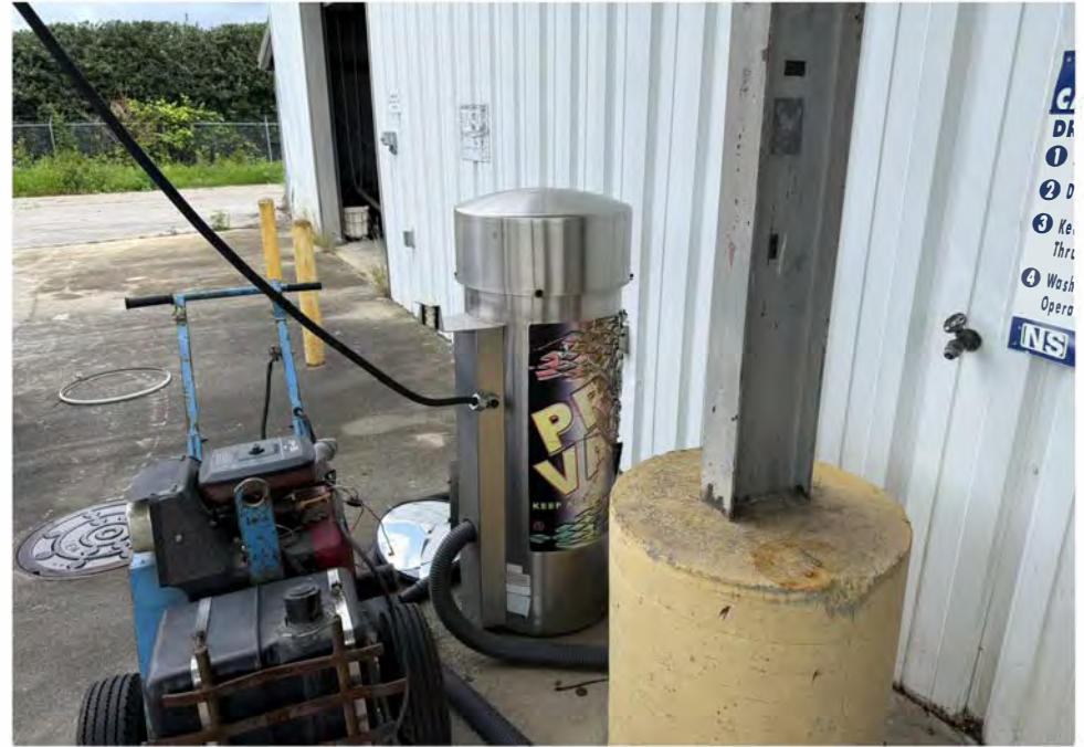
30> Air compressor at wash bay door
